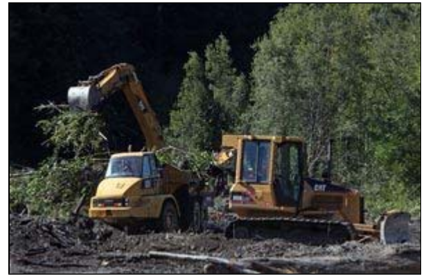
STEVE RINGMAN / THE SEATTLE TIMES Workers are taking out alders on a delta of sediment, clearing the way for a pilot channel to redirect the Elwha's flow.
