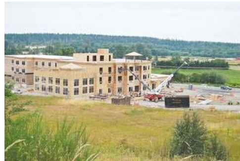
The Holiday Inn Express construction site greets travelers heading westbound into Sequim on U.S. Highway 101. The 77-room hotel and conference center is expected to open in November, with roof gardens, a swimming pool and convention facilities for up to 250.
